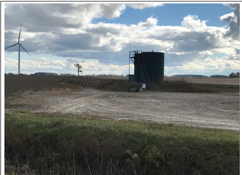
Photo 17 Silos and dispensing equipment observed at Lot 23, Concession 5, Romney.
