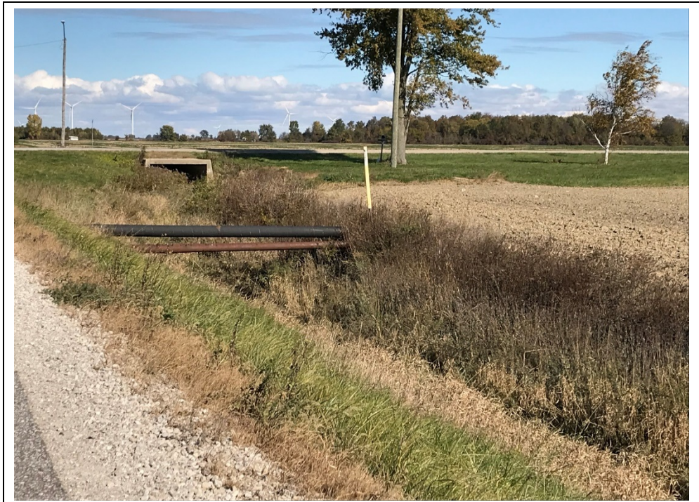
Photo 13 Exposed pipeline near Lot 1, south side of Middle Road, Tilbury West.
