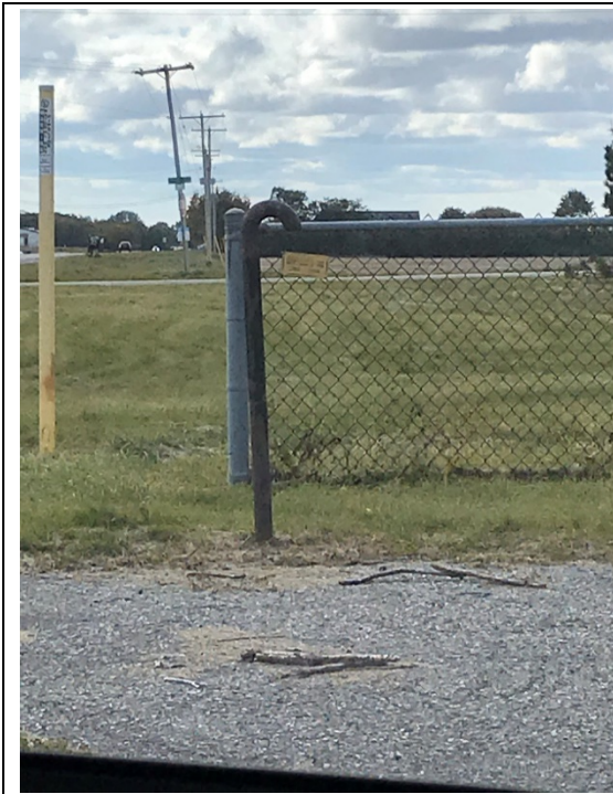
Photo 21 Vent pipe observed at 4495 Talbot Trail (PSOC 11).
