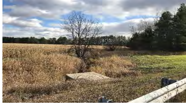
Plate 22: [E] Boundary Road culvert; Area beyond disturbed ROW and channelized creek requires Stage 2
