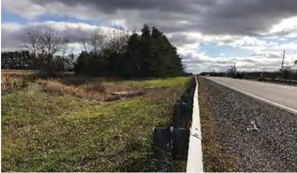
Plate 21: [SE] Boundary Road; Area beyond disturbed ROW and channelized creek requires Stage 2
