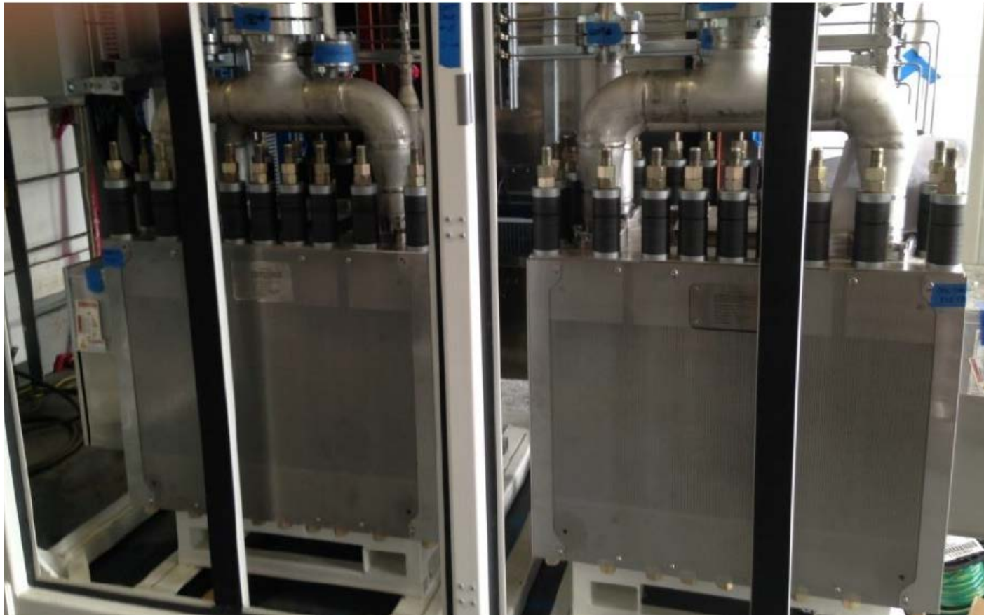
Source Image: Two Hydrogenics 1.25 MW electrolyser stacks installed at Markham Energy Storage Facility
