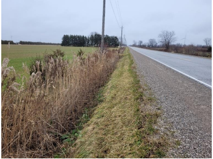
Photo 60: Steeply ditched ROW, facing east
