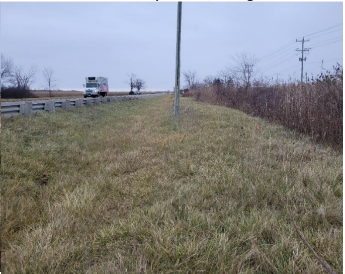
Photo 30: Ditched, built up disturbed ROW between municipal road and old rail line, facing east
