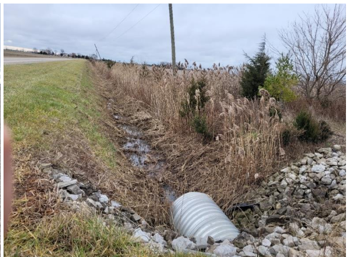
Photo 82: Disturbed ROW, deeply ditched with culvert, facing east
