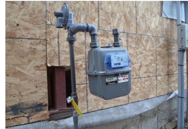
Figure 1 – Swing Joint Meter Set
