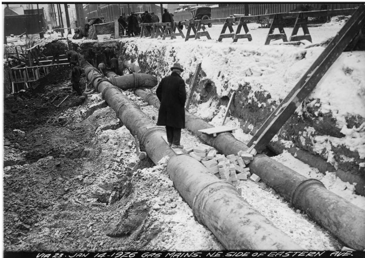
Plate 3: Example of deep excavation during the construction of gas mains on Eastern Avenue, 1926 (City of Toronto 2018b)
