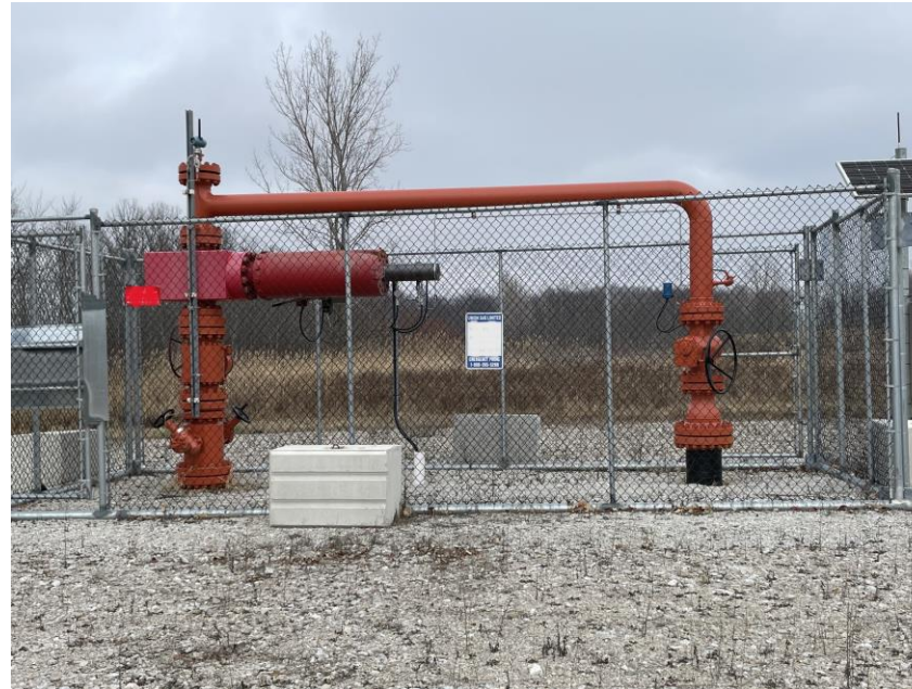
Image 1. Typical Injection – Withdrawal Well Wellhead
