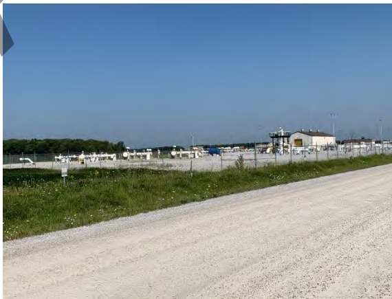
Photo 24: View of existing Enbridge infrastructure within the study area, facing northwest
