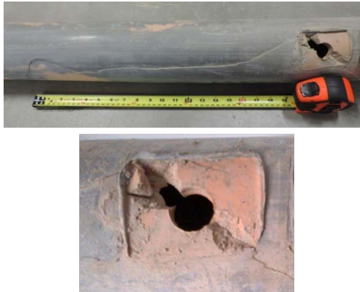
Figure 5.2-33: Rapid Crack Propagation on Aldyl A Pipe from Saddle Tee Fusion (Mississauga, ON)
