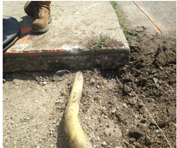
Figure 5.2-5: Shallow and Embedded Gas Main due to Road Grade Change
