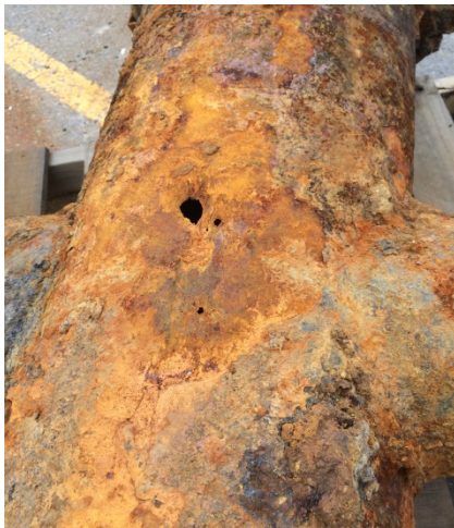
Figure 5.2-16: Multiple Leaks due to Severe Corrosion on Vintage NPS 12 Gas Main
