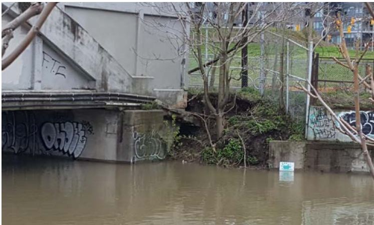
Figure 5.2-19: NPS 30 Pipe Bridge Westerly Abutment Undermining
