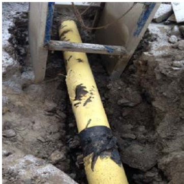
Figure 5.2-25: Gouges and dents due to latent damages
