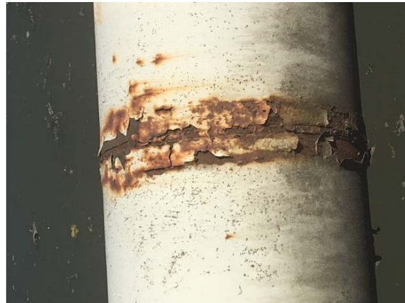
Figure 5.2-23: NPS 20 Pipe Crossing Exhibiting Corrosion
