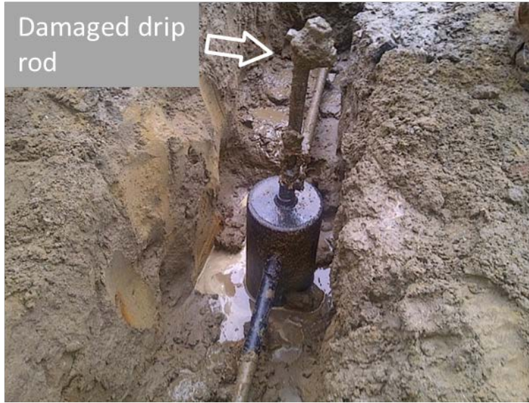
Figure 5.2-9: Damaged Drip Rod on Vintage NPS 2 Gas Main
