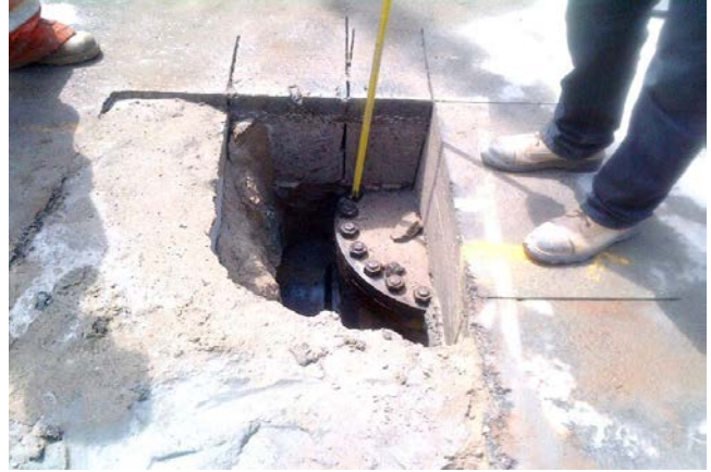
Figure 5.2-22: NPS 20 KOL Shallow Cover due to Road Grade Changes
