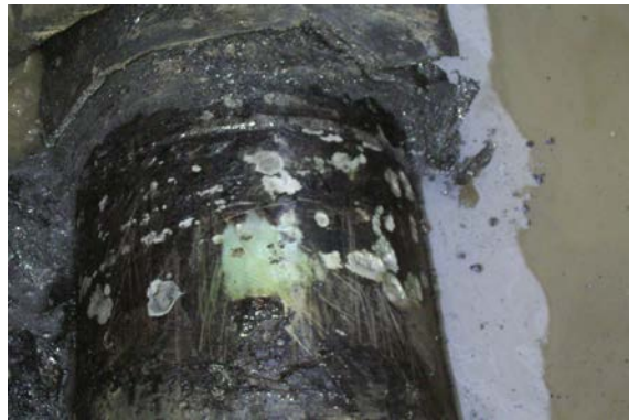
Figure 5.2-24: Multiple corrosion sites on NPS 12 St. Laurent XHP
