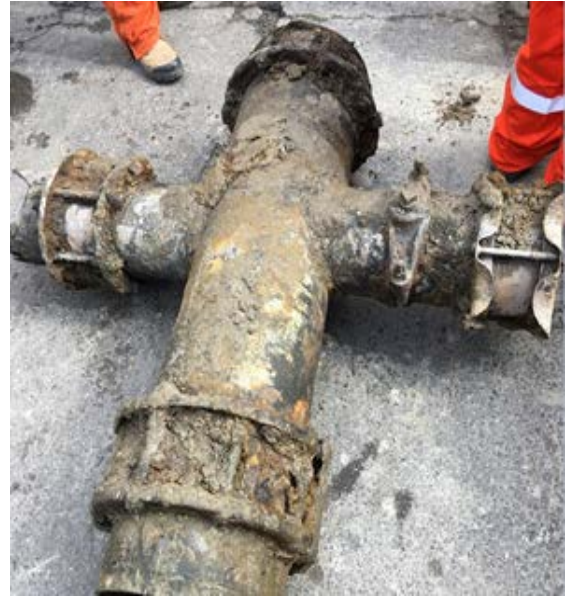
Figure 5.2-15: Shallow and Embedded Gas Main due to Road Grade Change
