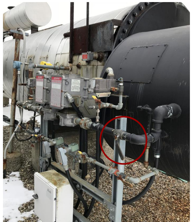
Figure 5: Valve used to throttle pressure to inlet of burners
